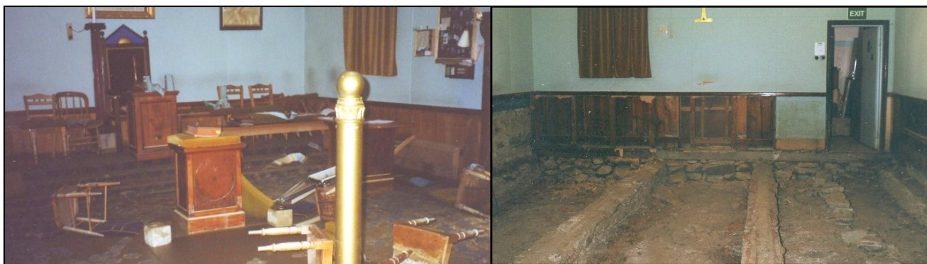
Left, interior of the Lodge room and, right, the exposed floor bearers
