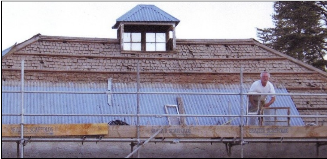
The roofing was removed, exposing the original shingles. The 1871 iron was then re-nailed in its former position.
